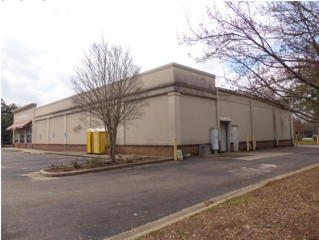
3. View southwest to the east (left) and north (right) elevations of the existing building on the property
