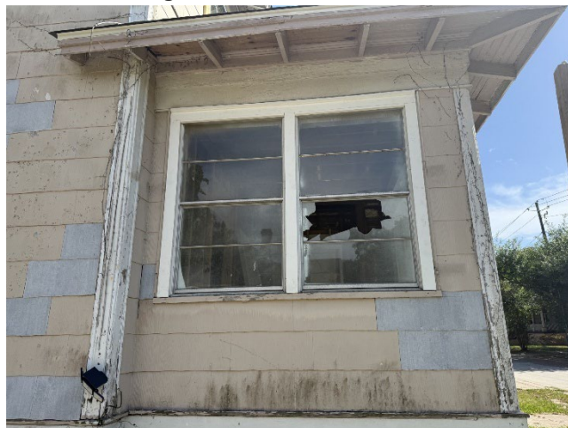
6. View of extant metal window on the north elevation of the enclosed porch.
