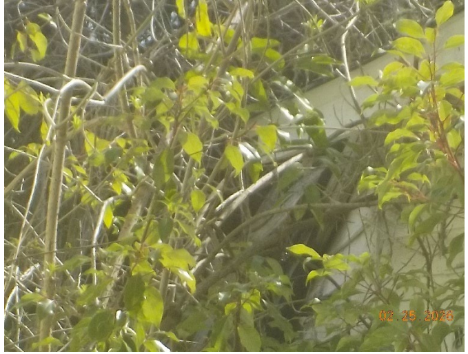
8. View of damage to east elevation (taken by Municipal Enforcement February 2026)
