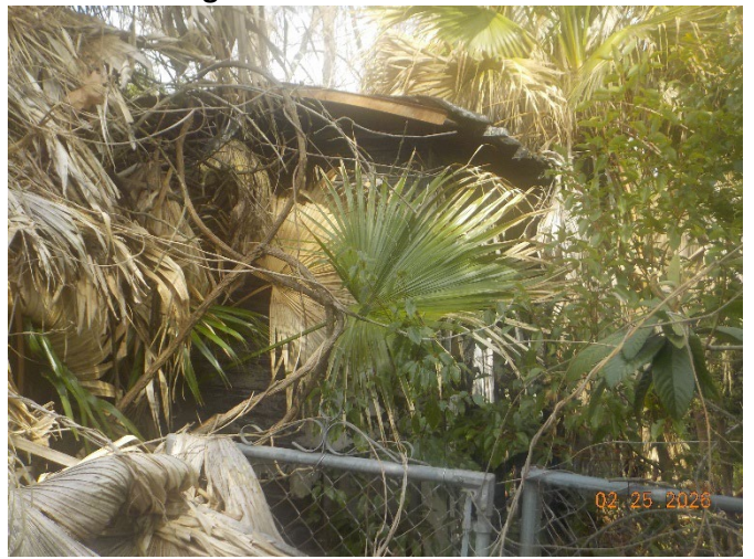
6. View of damage to east elevation (taken by Municipal Enforcement February 2026)
