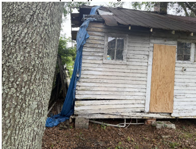
View of damage to west elevation, looking N
