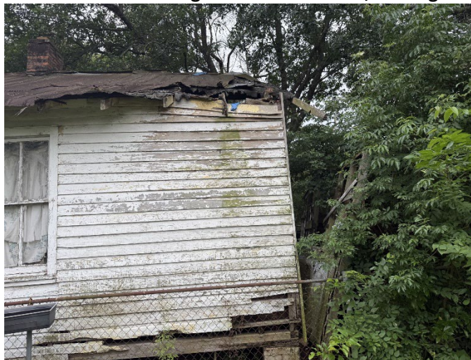
5. View of damage to west elevation, looking S
