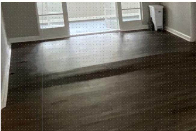
5. Bowing of the floor in interior living space, looking east.
