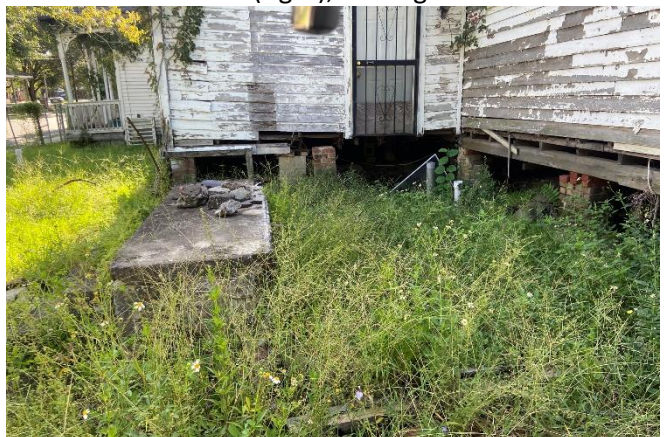
6. Sill plate of c. 1942 addition visibly bowing over insufficient brick piers
