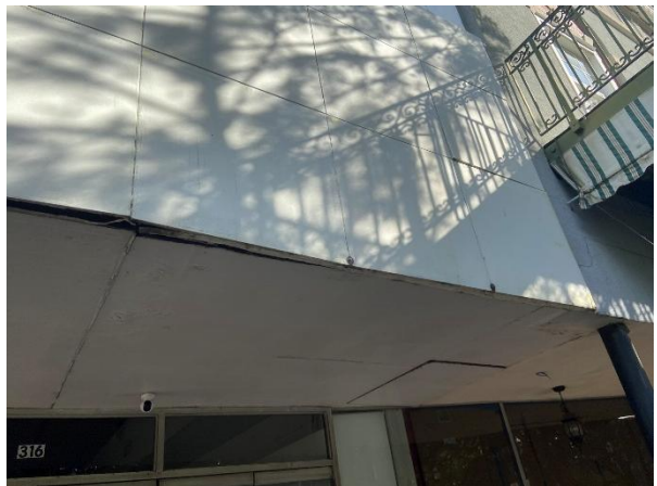
12. 316-318 Dauphin, displacement and previous repairs of existing aluminum cladding
