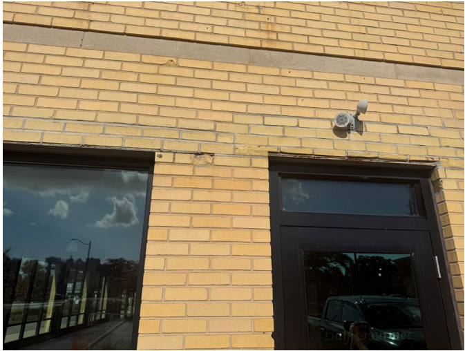
13. Detail of damaged and infill brick on south elevation
