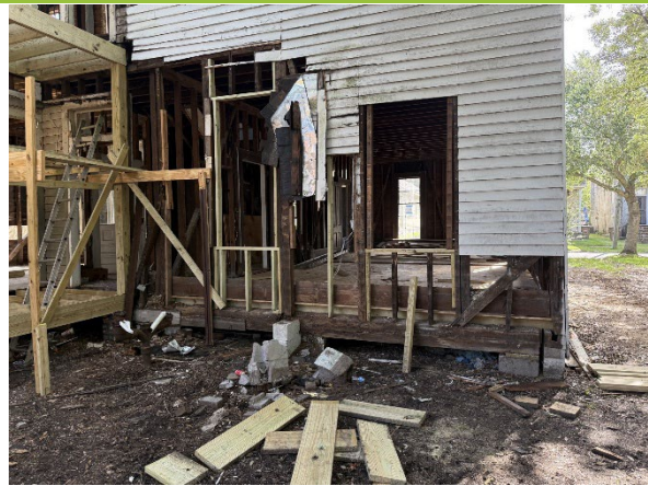
8. View of damaged clapboard siding on the west elevation.
