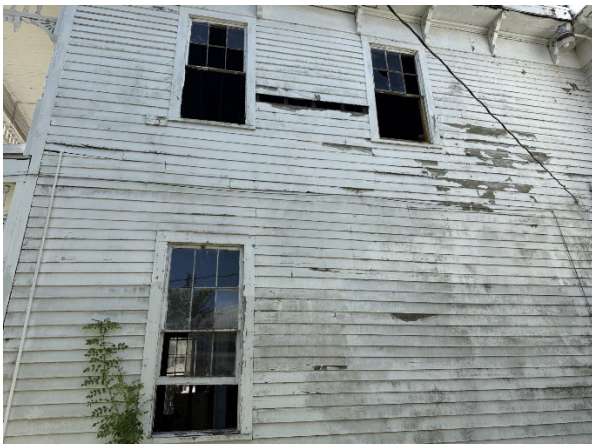
5. View of damaged clapboard siding on the north elevation.
