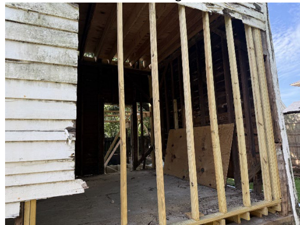
6. View of missing clapboard siding on the north elevation of the rear wing.
