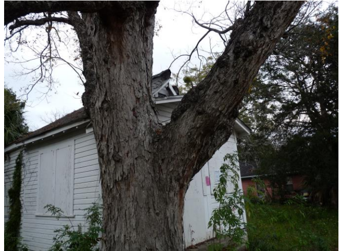
2. View of roof damage on front gable
