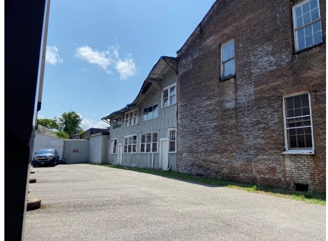
8. View northwest to frame and metal enclosure of double gallery at rear wing
