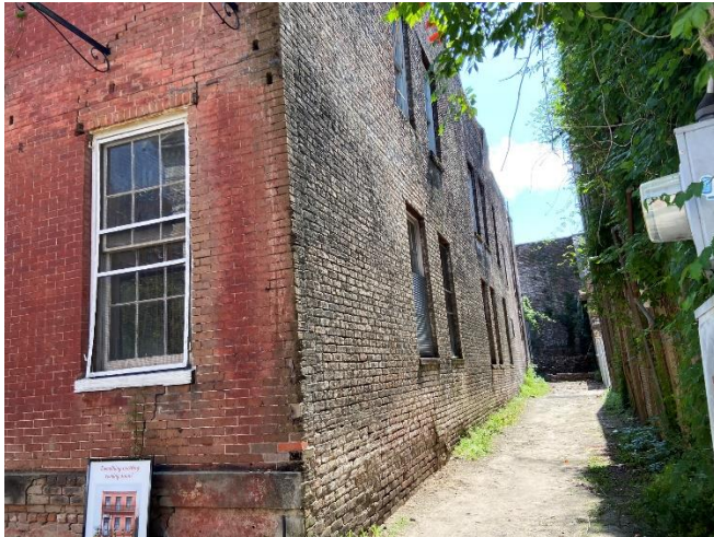
9. view west-southwest to north elevation of subject property; note precarious condition of brick wall
