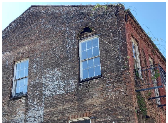
6. View north-northwest to area of missing bricks over window on south elevation
