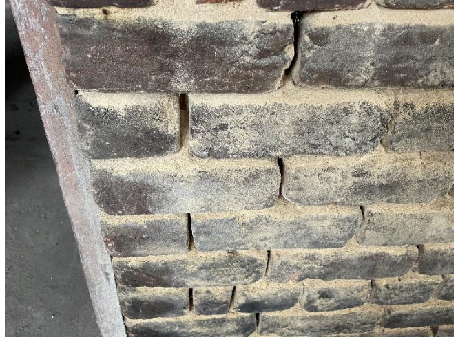
2. example of deteriorated mortar in south wall of rear wing
