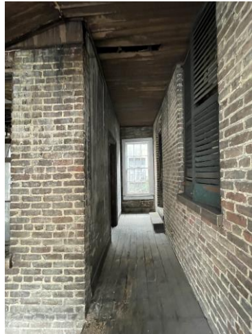
4. View north into space between front block of house and rear wing (shown as frame porch on Sanborn maps)
