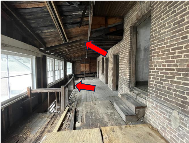
3. View west along south elevation, 2nd floor porch, rear wing; note later roof extension and stairs (left)
