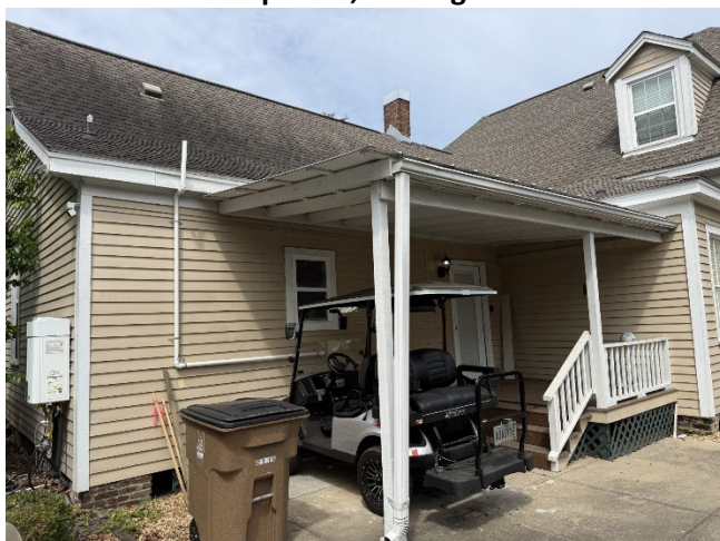
4. Subject shed roof projection on the east elevation proposed for demolition, looking west.
