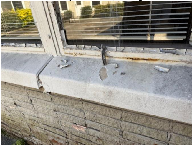
11. Detail of window deterioration
