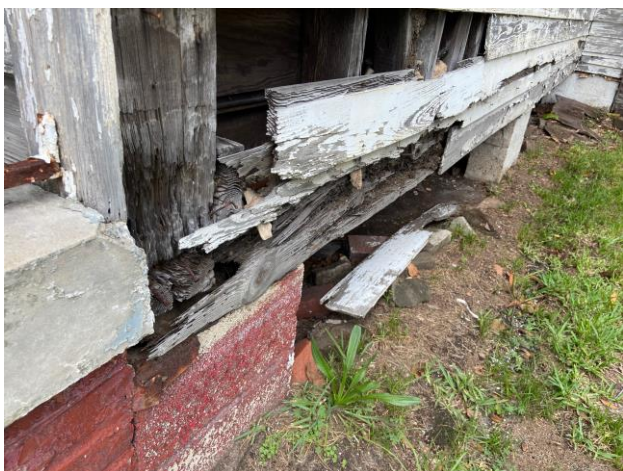
5. Detail of deterioration
