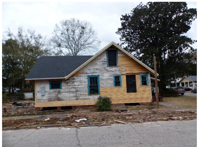
6. North elevation, looking south. New window opening shown at former location of demolished chimney.
