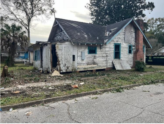
7. North elevation prior to removal of chimney and rear addition (photo provided by applicant)
