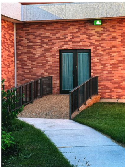
5. Entry door to be replaced (and awning installed above) on west projection, view to south.
