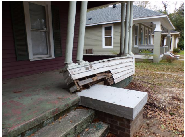
2. Detail: damaged porch columns and knee wall, looking southeast
