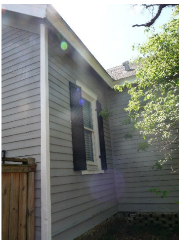
3. View of north elevation of east wing, looking W. The window would be removed, and the proposed porch would span this elevation.
