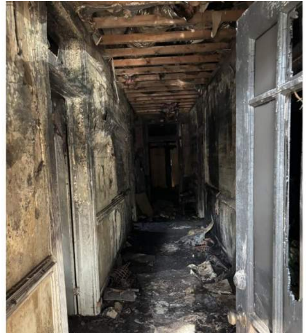
5. Interior fire damage, view east from front door
